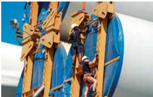
Hooking to tower sections. Work carried out at height. Personal safety is paramount.
